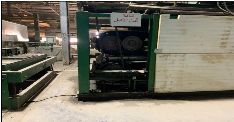
Picture (3) of one of the malfunctioning machines in the metal industrial facility for the public sector in Al-Nasr Company in Taji District
